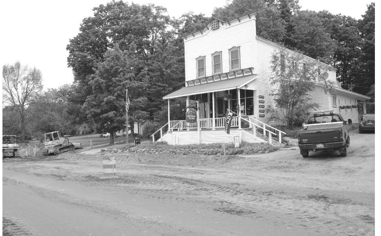
The road construction made it difficult to get to the Horton Bay General Store.
